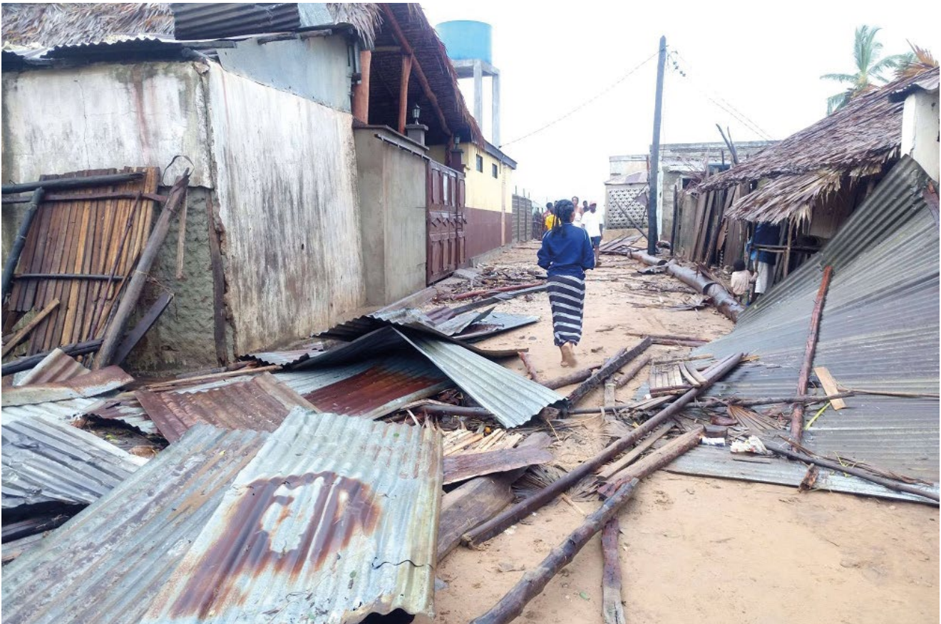
Tropical cyclone damage, Madagascar. Image: Malagasy Red Cross
